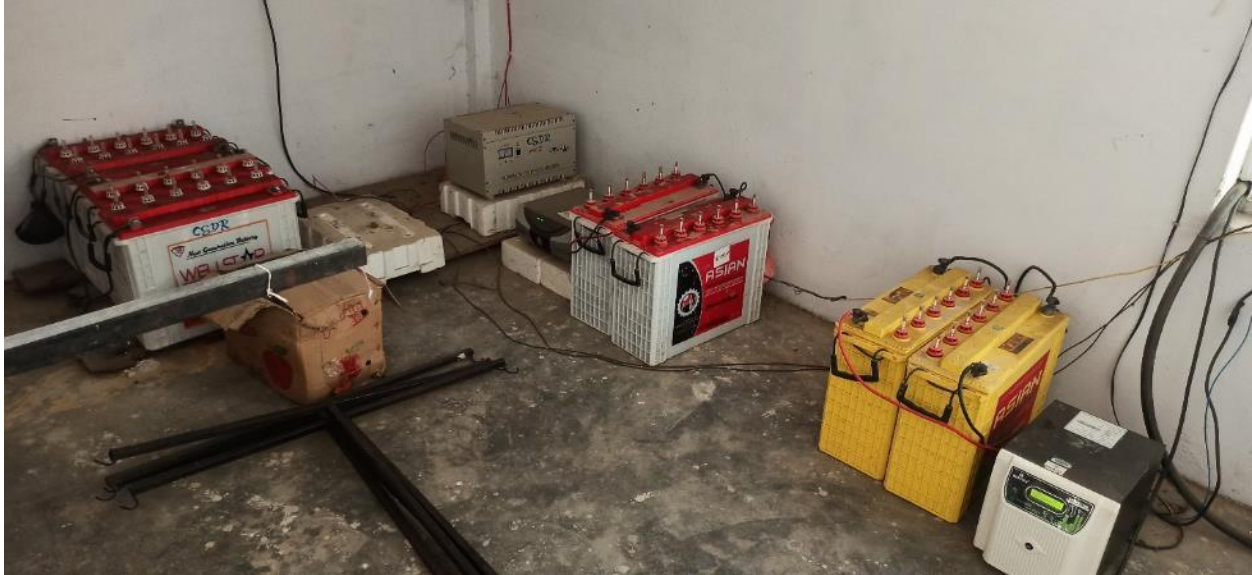
Figure 17: Battery and inverter backup in Rajapur, Bardiya
