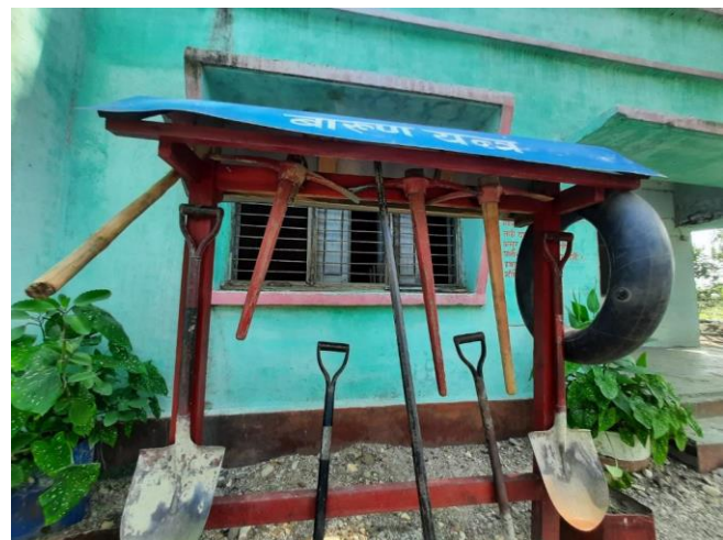
Figure 20: Open access firefighting equipment in Chandrapur, Rautahat
