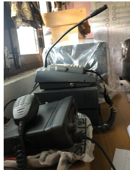
Figure 18: VHF, HF and telecommunication devices at PEOC, Kaski
